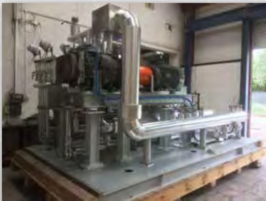
Nitrogen Start-up Blower
