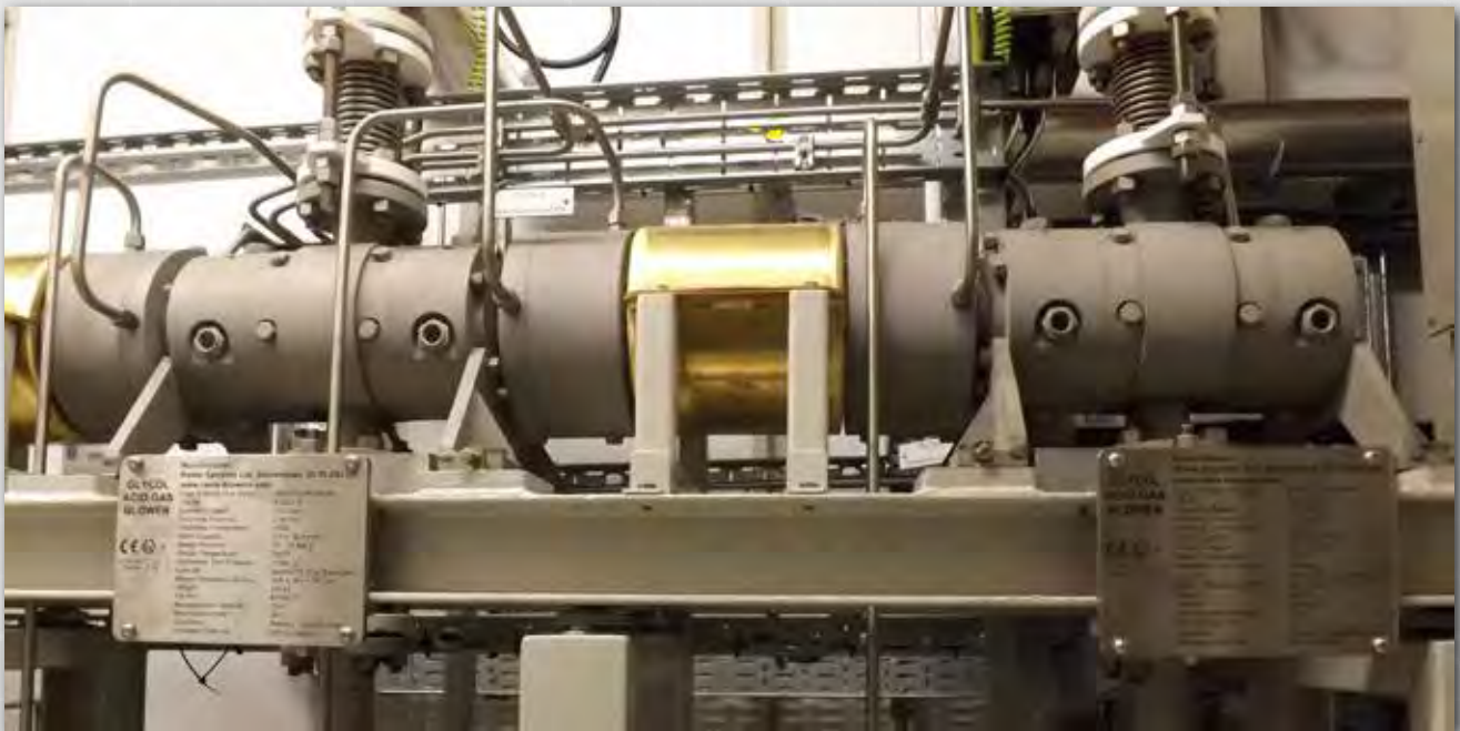
Glycol Acid-gas Blower
