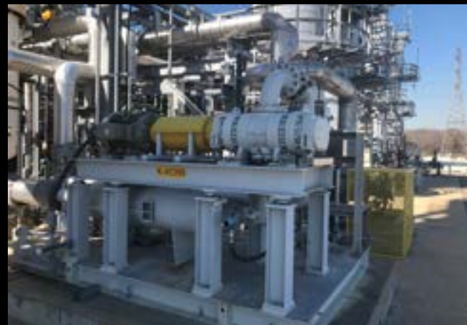
Regeneration Gas Compressor Package
